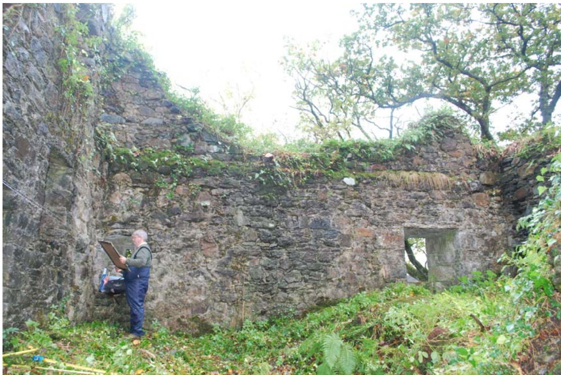
View to the S, Tom Addyman recording the interior elevations after elm, ivy and saplings removed.
